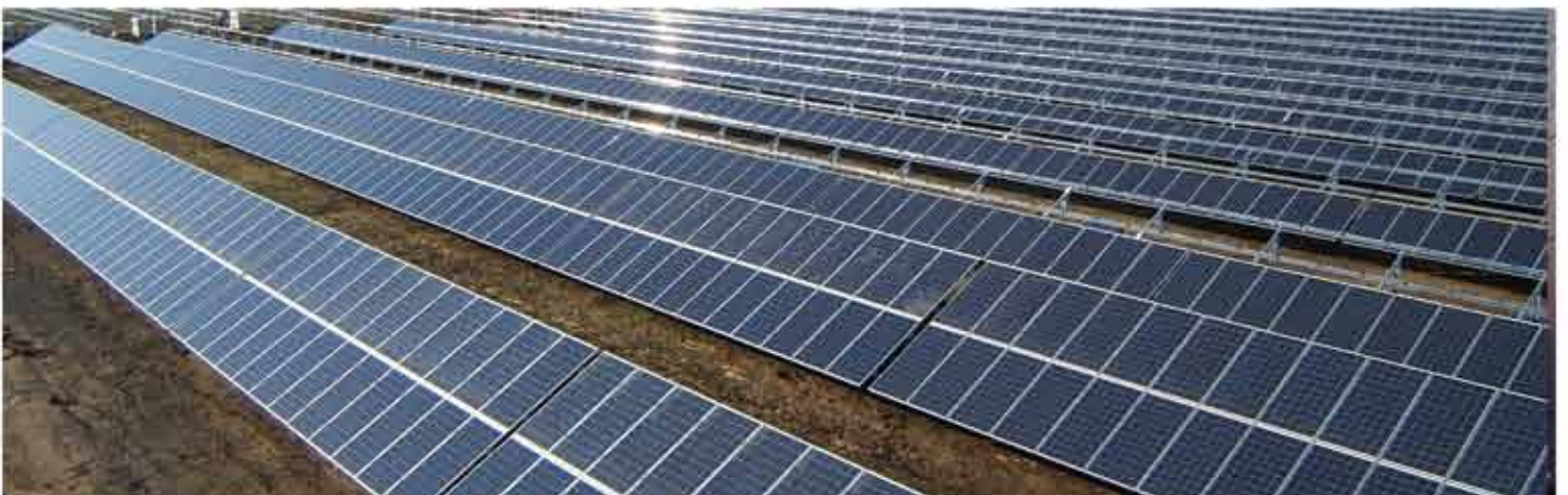
■ Solar Power Plant
